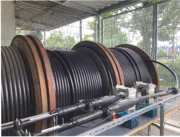
Figure 1: Test cable setup with three cables in the background, and two straight joints with connected high frequency current transformers in the foreground.
